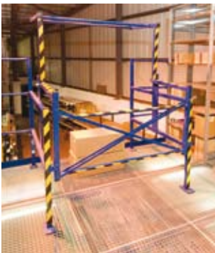
A pivoting safety barrier ensures the fence opening is guarded at all times
