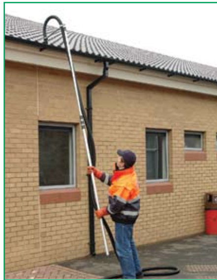
Figure 1 – This is an example of using suitable work equipment to avoid working at height
